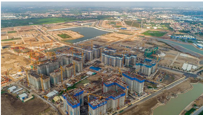
Figure 31: Ocean Park - First high-rise section could be ready for handover in FY20F
