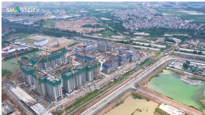
Figure 33: Smart City - Eight blocks of condos have finished foundation works and body construction up to the 12th floor
