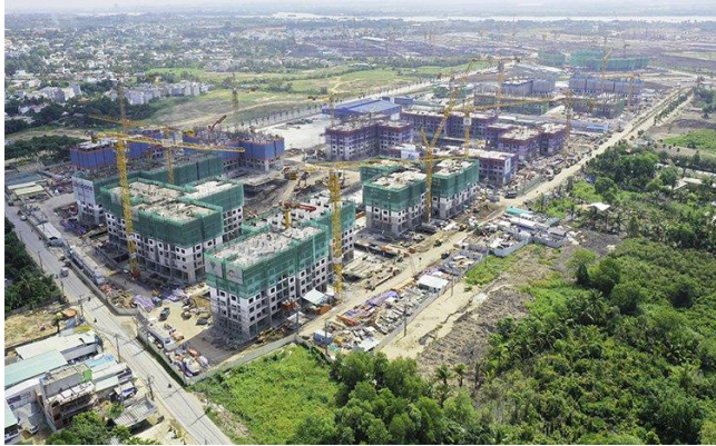
Figure 35: Grand Park – First condo section (17 blocks) has finish foundation works and body construction up to 21th floor
